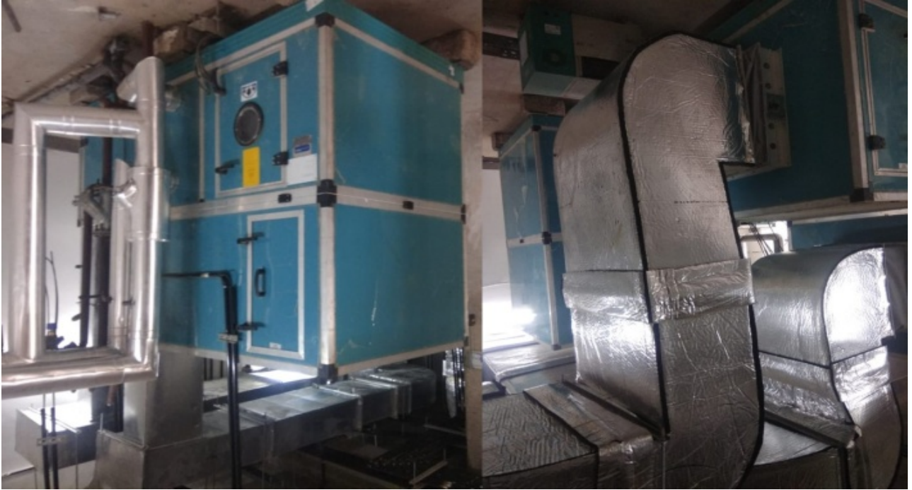
Installation of dedicated double skin AHU for Transplant OT's at D&T OT Block (1)
