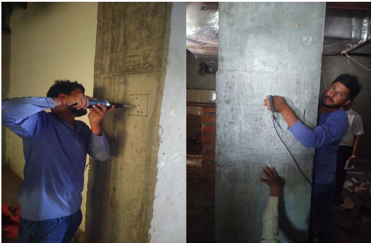
Non Destructive Test for Structural Elements of Building at Newly Constructed D&T OT Block
