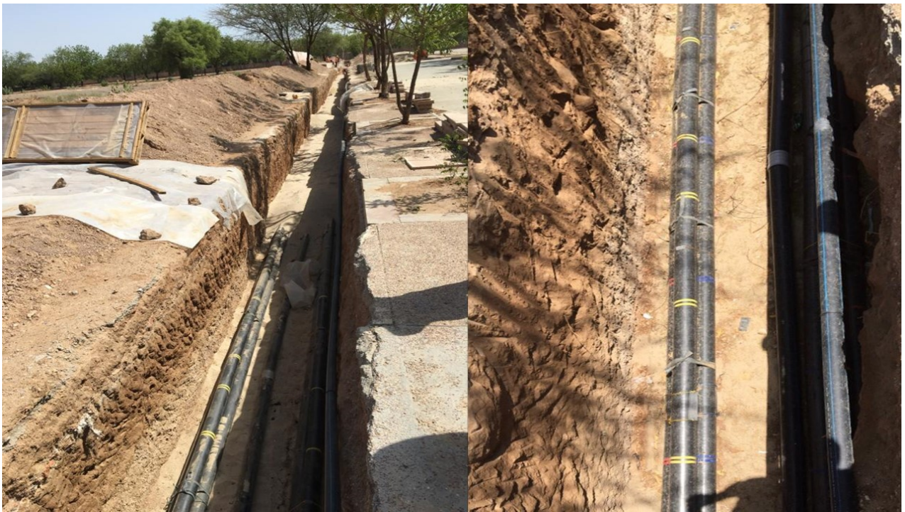
Over head to Under ground Laying work of 132 kV double circuit EHV Line
